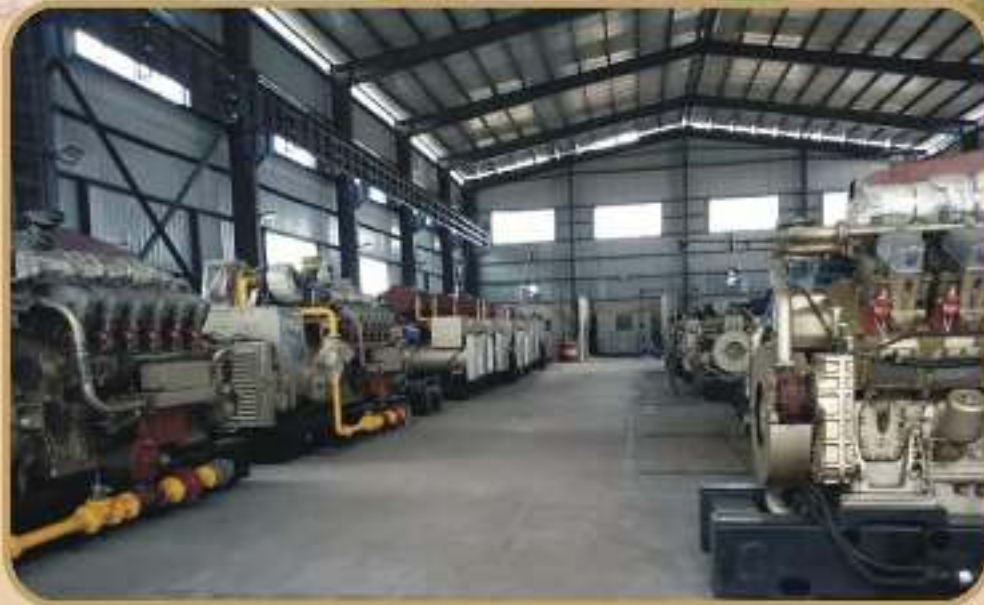
INSIDE VIEW OF OSSIOMO - POWER PROJECT
